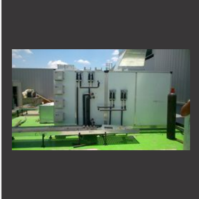
VRF Air Conditioning System
