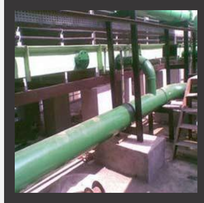
Condenser Water Piping Service
