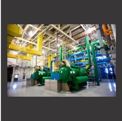
Chilled Water Piping Services
