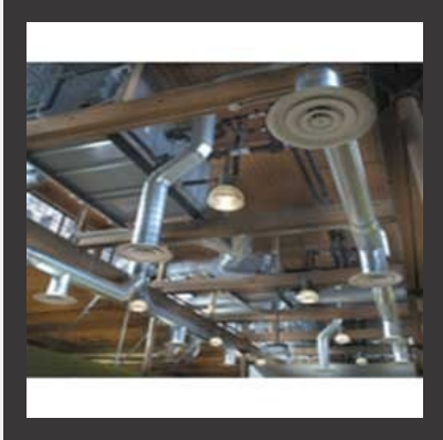
Process Ventilation System
